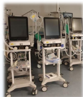
Installed NKV-550 ventilators in Scotland in Jun. 2020
